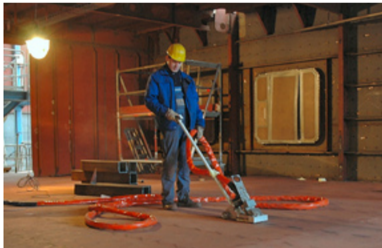
Clean, safe, comfortable. Induction fairing drastically improves the quality and the working environment. Nitrous gases, for example, are radically reduced.
