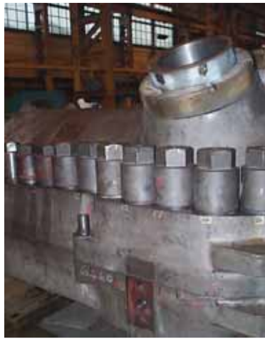
Waiting for induction—a typical bolt assembly at a power station.
