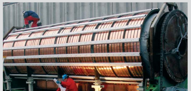
A specially designed EFD Induction coil being prepared for installation at a customer in Norway.
