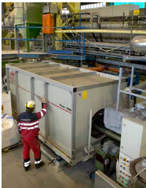
An example of induction pre-heating: the pipe is being heated prior to receiving an anti-corrosive coating.
